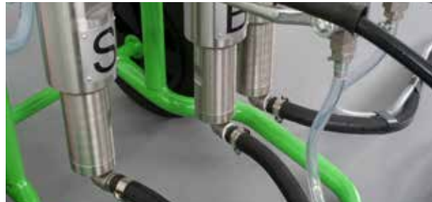
Material intake hoses
